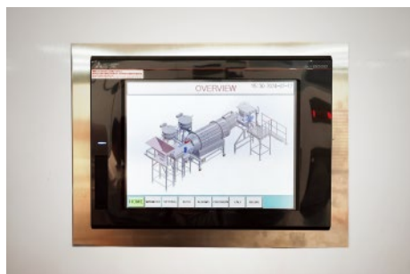
Despite the steep learning curve, the engineering team at SV Agri have put a lot of effort and diligence in creating their control systems.
